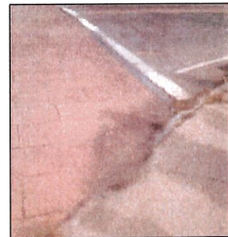
Signs of ponding on the crosswalk
